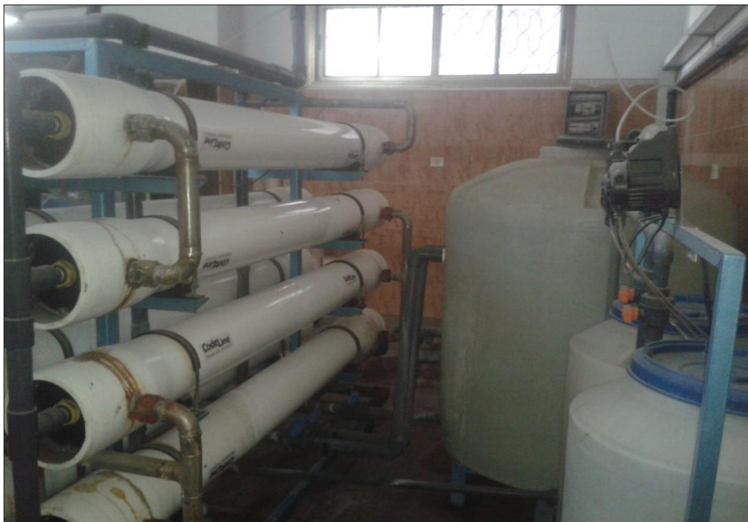
Figure (3.12): Pumping and storage in Al Manar plant
